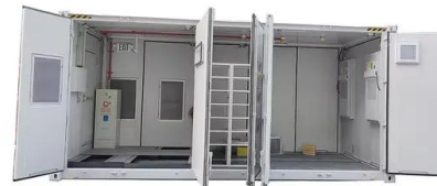
1075KW HH ESS
