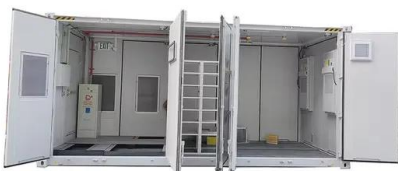
1075KW HH ESS
