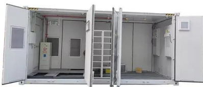
1075KW HH ESS
