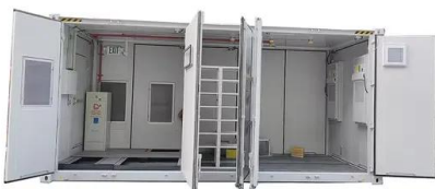
1075KW HH ESS
