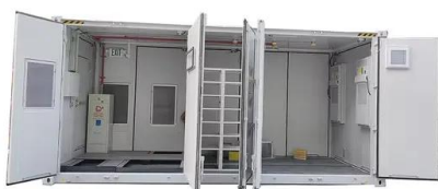
1075KW HH ESS
