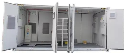
1075KW HH ESS
